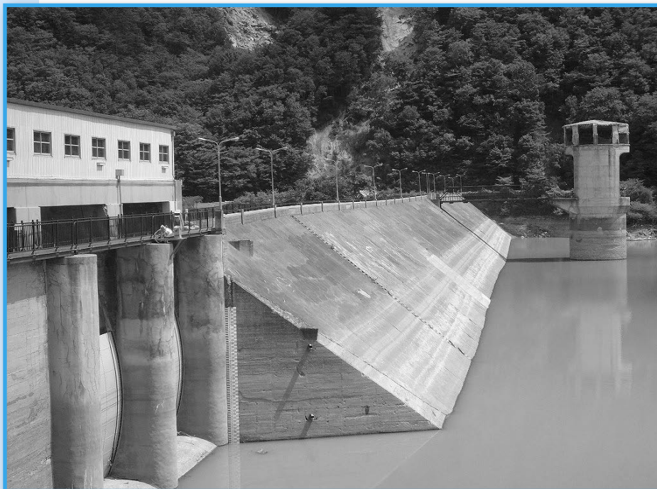
Photo-4 Concrete Face after the Earthquake
