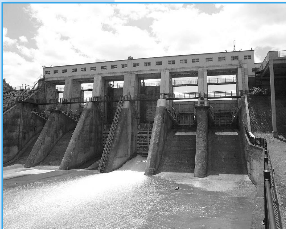
Photo-5 Spillway after the Earthquake
