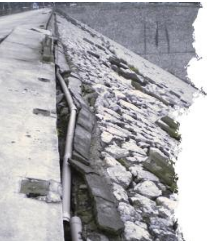
Fig. 3: Damage at crest of Zipingpu CFRD (downstream face)
