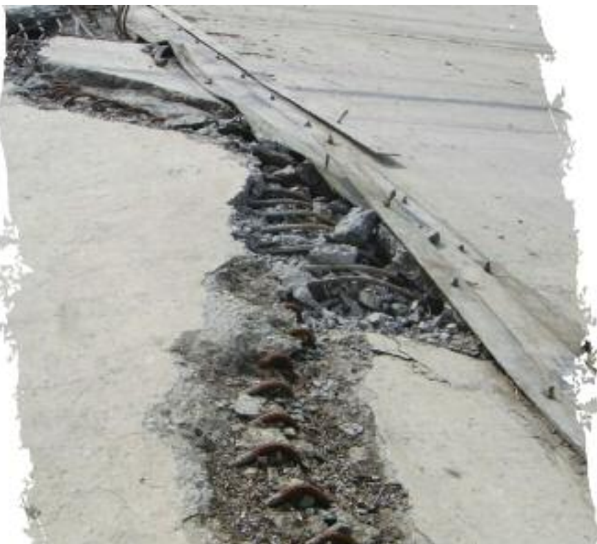
Fig. 4: Damage at crest of Zipingpu CFRD (downstream face)
